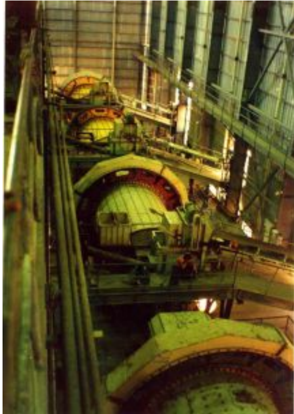
Ball mill for ore grinding
